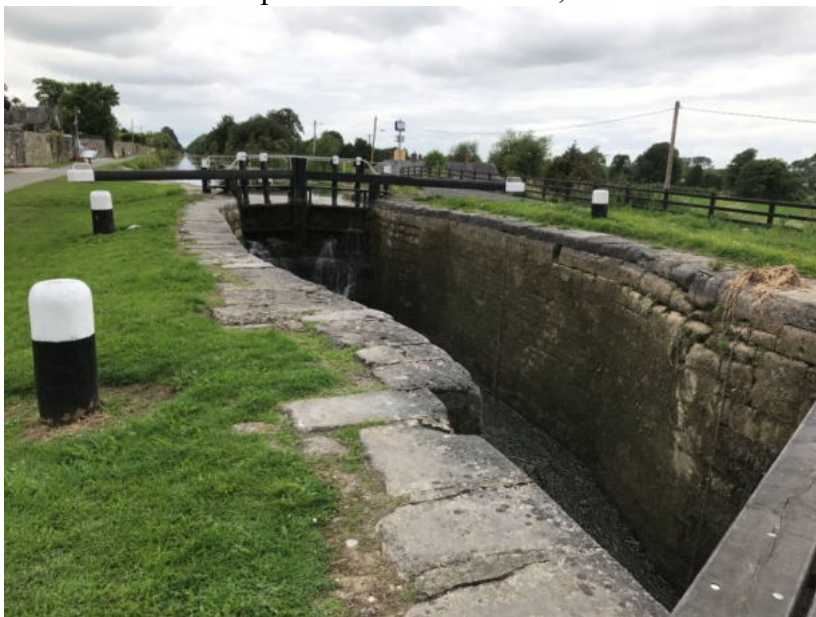
The upper chamber of the 13th Lock at Lyons was built to Omer's specified width of 20ft; the entrances were subsequently reduced to 16ft
